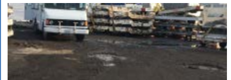
2020 Airfield Pavement Replacement Project – Distressed Asphalt Concrete Pavement.
