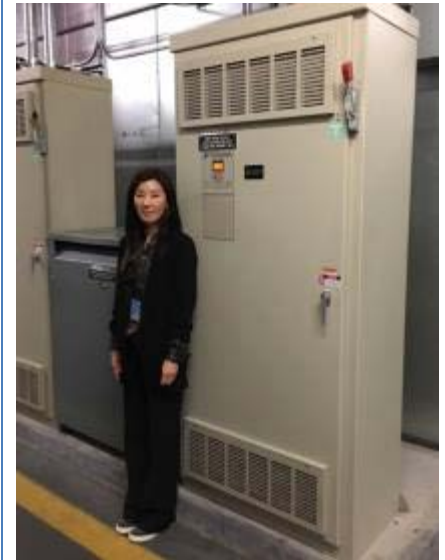
VFD Powering a 350 HP motor
