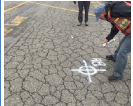
2019 Airfield Pavement Replacement Project – Distressed Asphalt Concrete Pavement.
